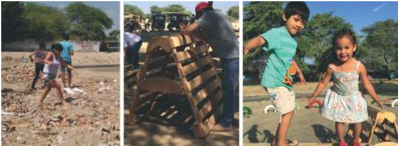
Figure 5. Part of the process of execution of Santa Julia Park. Source: Photography taken by the authors.
