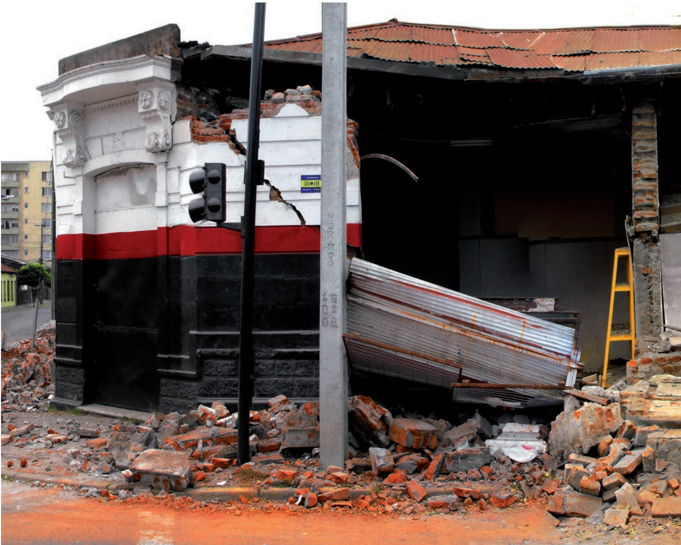
Figura 8 A 10 días del terremoto. Esquina calles Colo Colo y Cruz. Antigua edificación de fachada continua, estructurada a base de ladrillo que albergaba recintos comerciales. / Ten days after the earthquake. Corner of Colo-Colo and Cruz. Old brick street front building that used to house mainly commercial dependencies.
