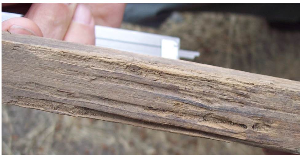
Figure 3. Termite attack on untreated radiata pine wood control stake detected during year-3 inspection trip.
