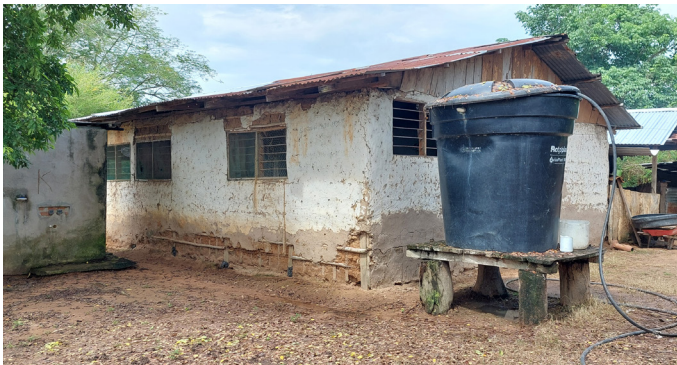
Figure 14. Traditional rural house in embedded adobe, La Zapatosa. Source: Preparation by the authors.
