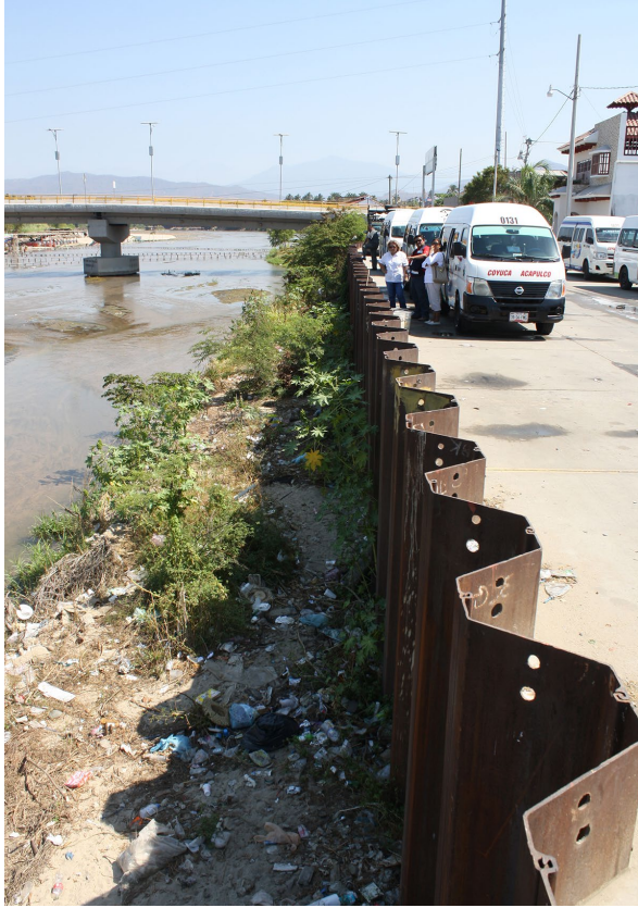
Figure 3. Protection curtain and Coyuca I Bridge in April 2017. Source: Photograph courtesy of the Coyuca Climate Resilient Project.
